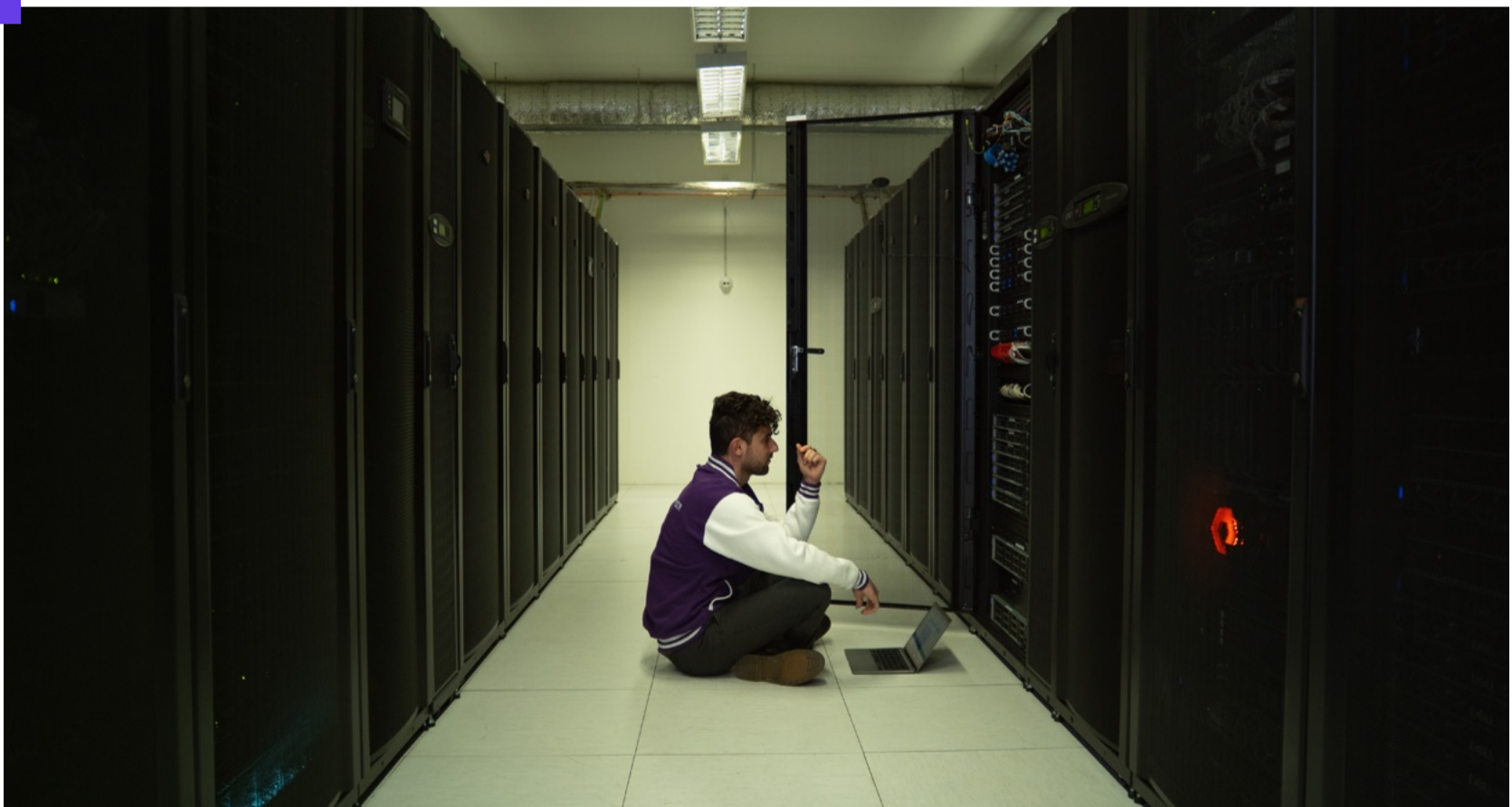
Hostinger - employee in data center
