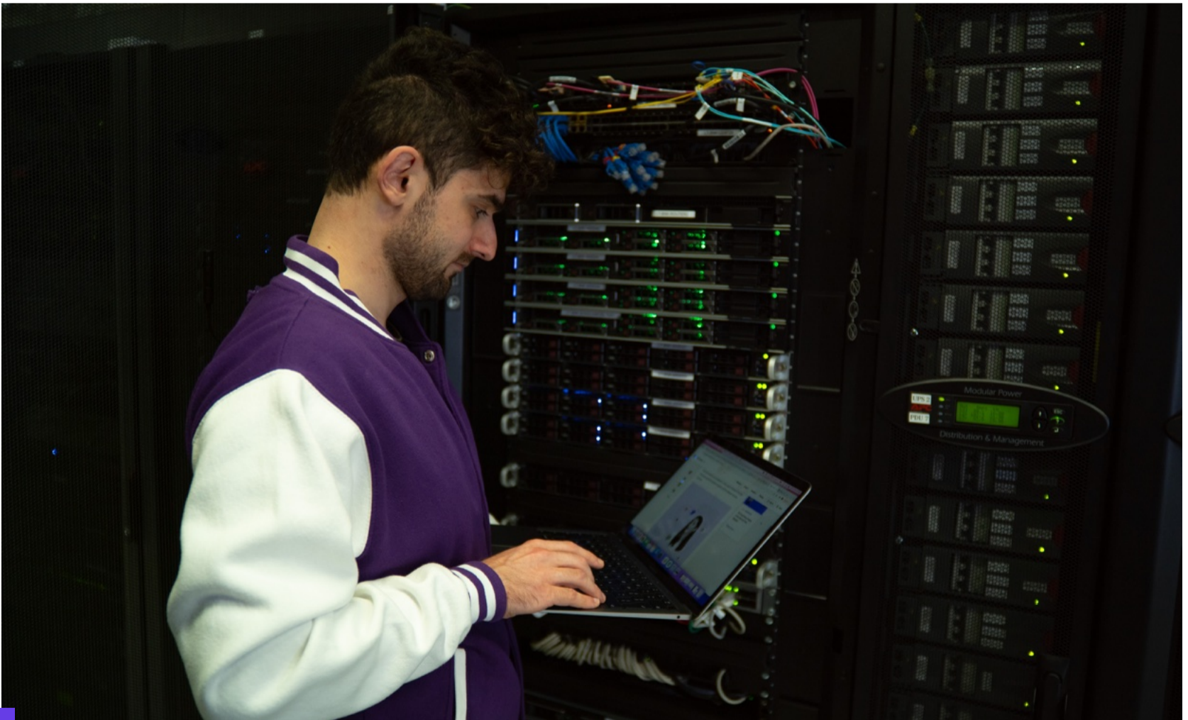
Hostinger – employee in data center
